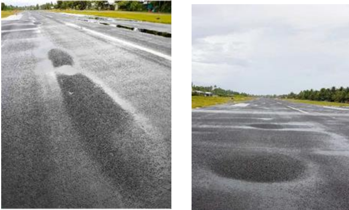
Figure 2: Blistering and depressions on runway
